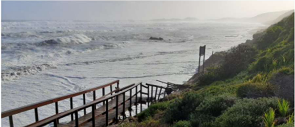
Fig.12. September 2023 storm surge, which washed away the Brenton on Sea beach walkway.
