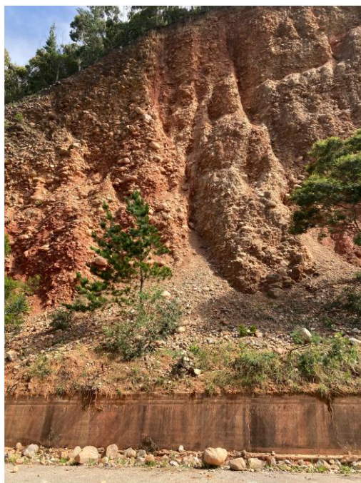
Fig 3: Photograph showing exposed unstable sandstone conglomerate above the DR1888 road to the west of portion 91/304, similar to the sandstone conglomerate on the Kaaimans Pass
