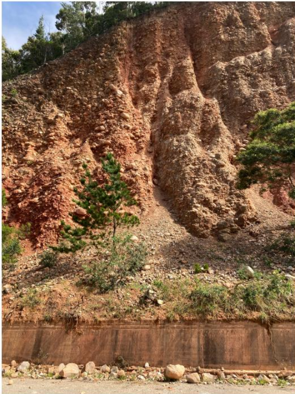
Fig. 5: Photograph showing exposed unstable sandstone conglomerate above the DR1888 road, immediately to the west of portion 91/304
